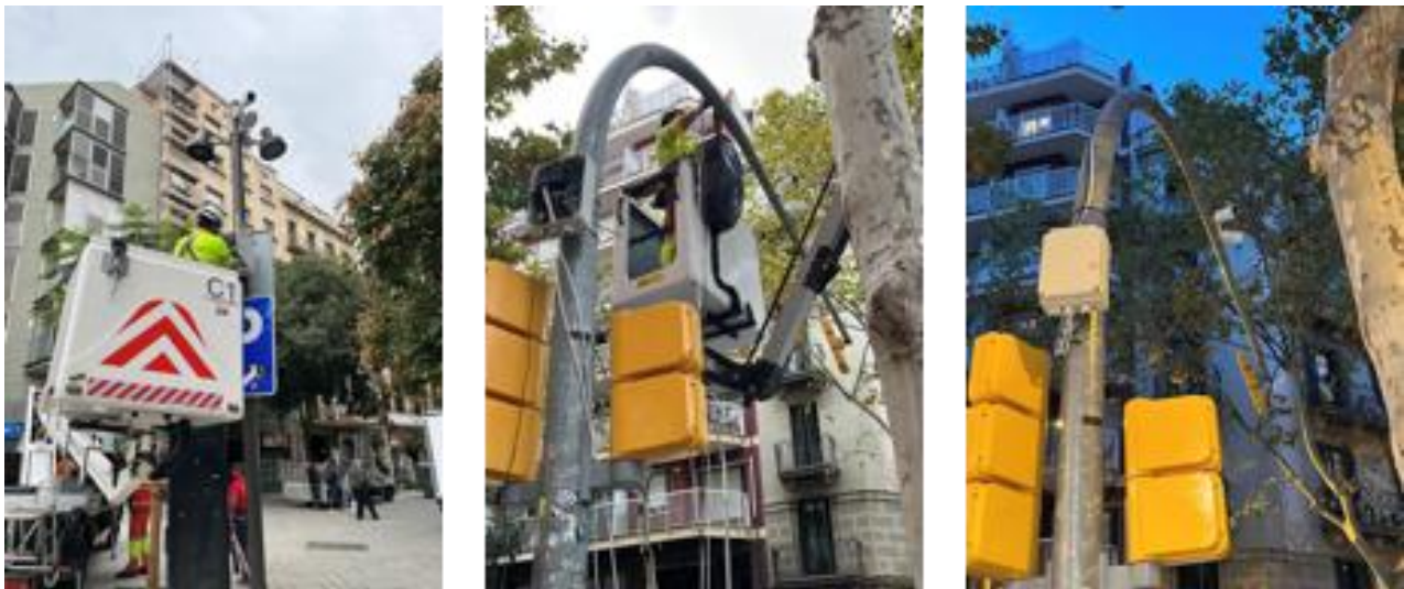
Figure 36 Camera installation in municipal light fixtures and traffic lights
