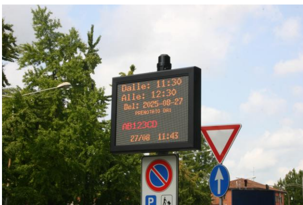
Figure 2 DISCOCURB Variable Message Signage
