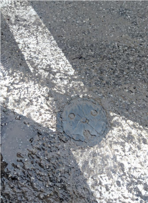
Figure 5. Remains of a mechanically damaged sensor on the surface of the bay (Narutowicza Street)
